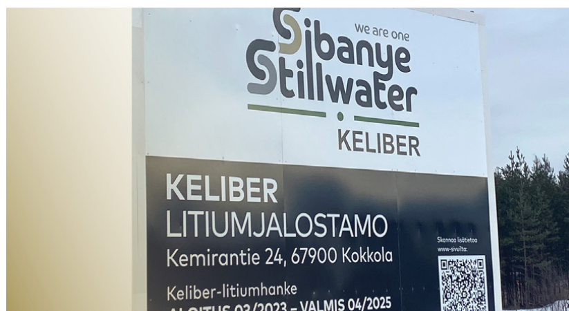
Branded sign at the construction site of the Keliber lithium refinery in Kokkola, Finland
